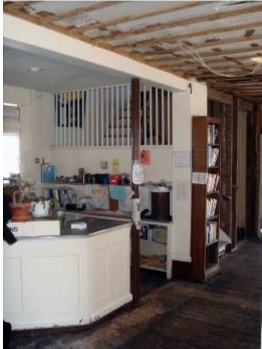
Ceiling damage due to flood
