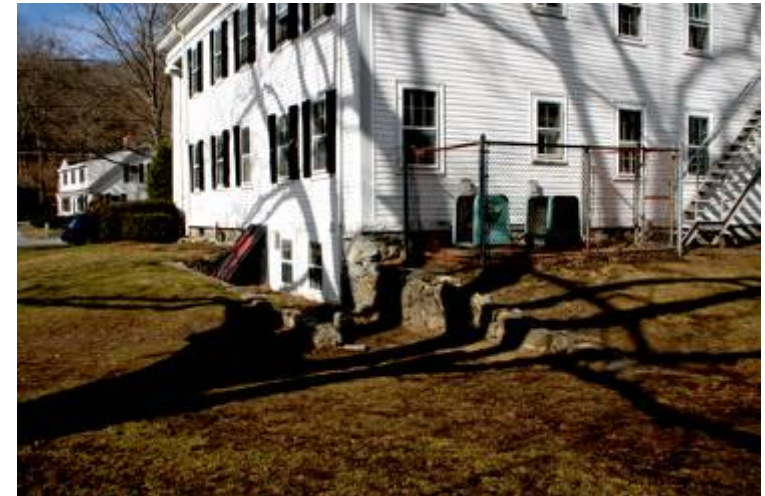
Exterior mechanical equipment
