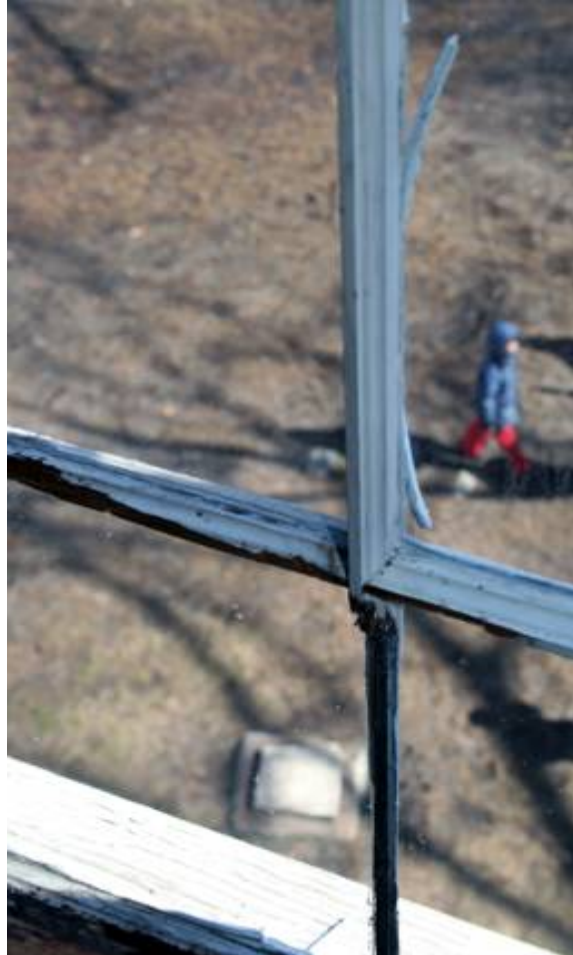
Attic window damage
